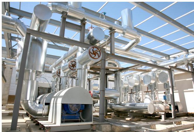
Fig. 2(b): Primary-Secondary Chilled Water Pumps
