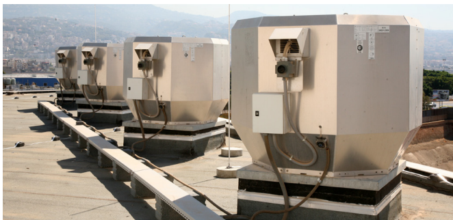
Fig. 5(a): 4 No. Systemair Smoke Extract Fan DWV 1000 D4-F400 for Cabin Crew Simulator Area
